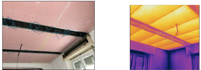
Fig. 1. Installation of the heating system (left) and thermography picture of the panels while working, by means of a thermoscanner (right)
