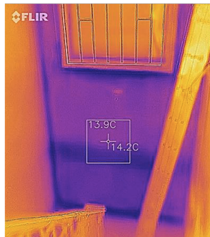
Fig. 2. Thermography of an external wall before the nanotechnology-based insulation.
