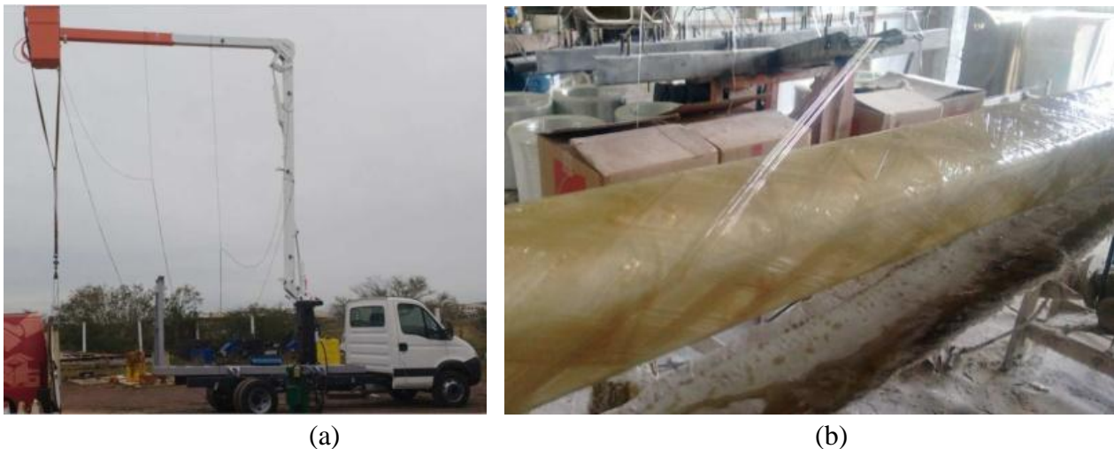
Figure 8. (a) Application of the GFRP and (b) detail of the manufacturing of the GFRP rod.
