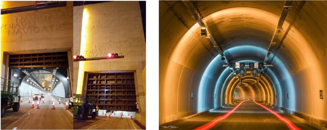
Figure 1. (a): Miami Tunnel with flood gates (Florida, USA); (b) Ovit Tunnel over 14 km long (Turkey)
