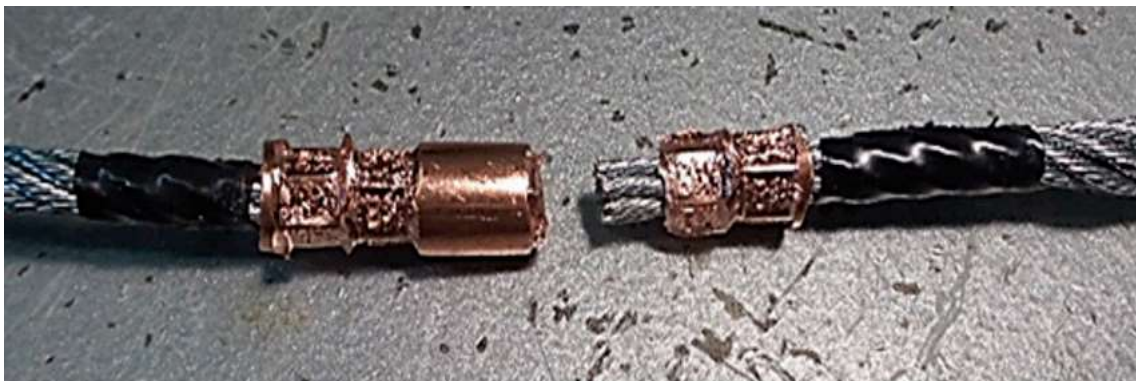
Figure 5. Breakage of the connector clamp, close of the variation in the resistant cross-section.
