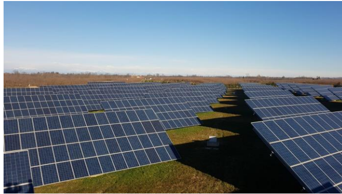
Fig. 4. PV generators of one of the ground-mounted systems under analysis
