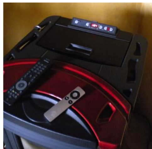
Fig. 4 - Wood stove connected to the controller.
