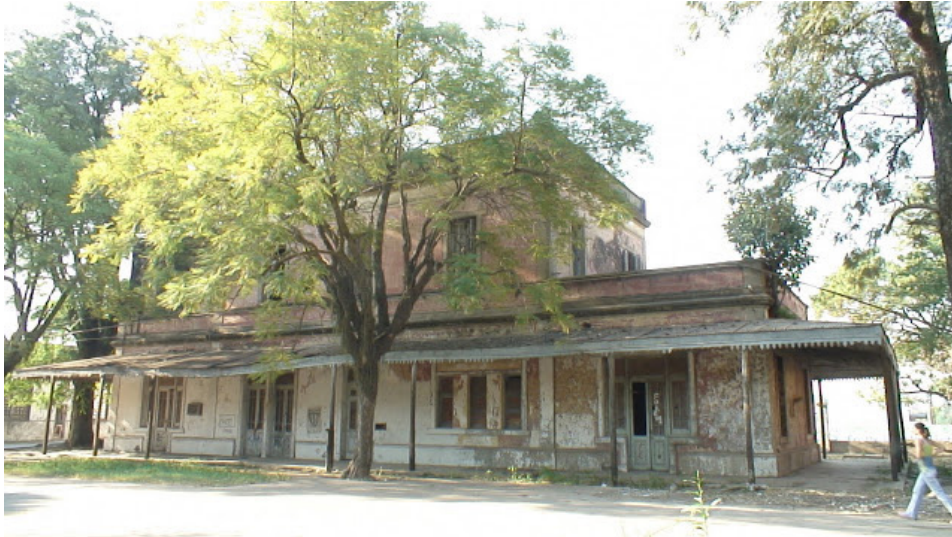
Fig. 7. "La Fabril" Headquarters building (2018). Many buildings are in poor condition, as the main office building; they still keep in place original building details of great interest.
