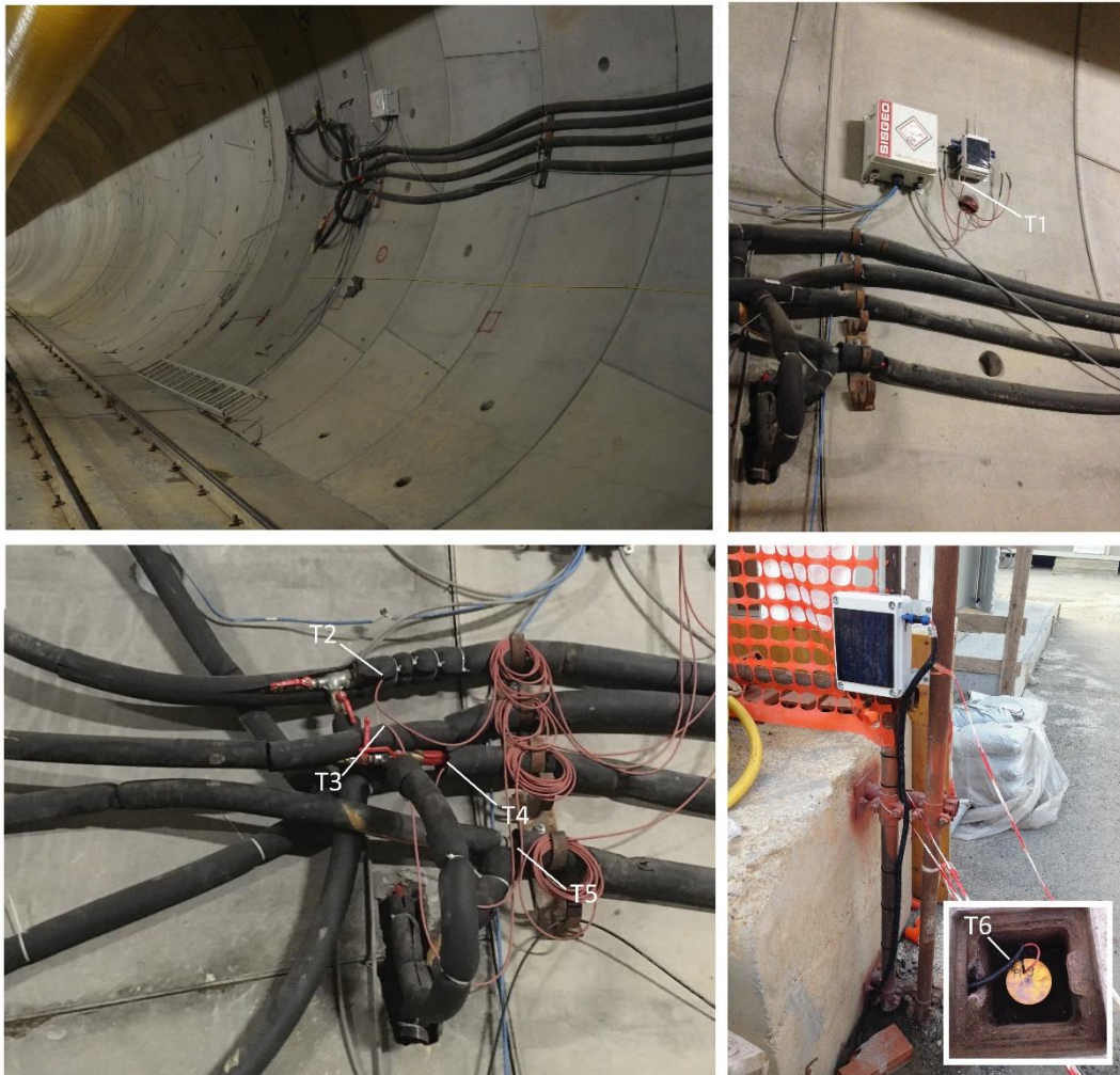
Figure 4.15: Location of the temperature probes.
