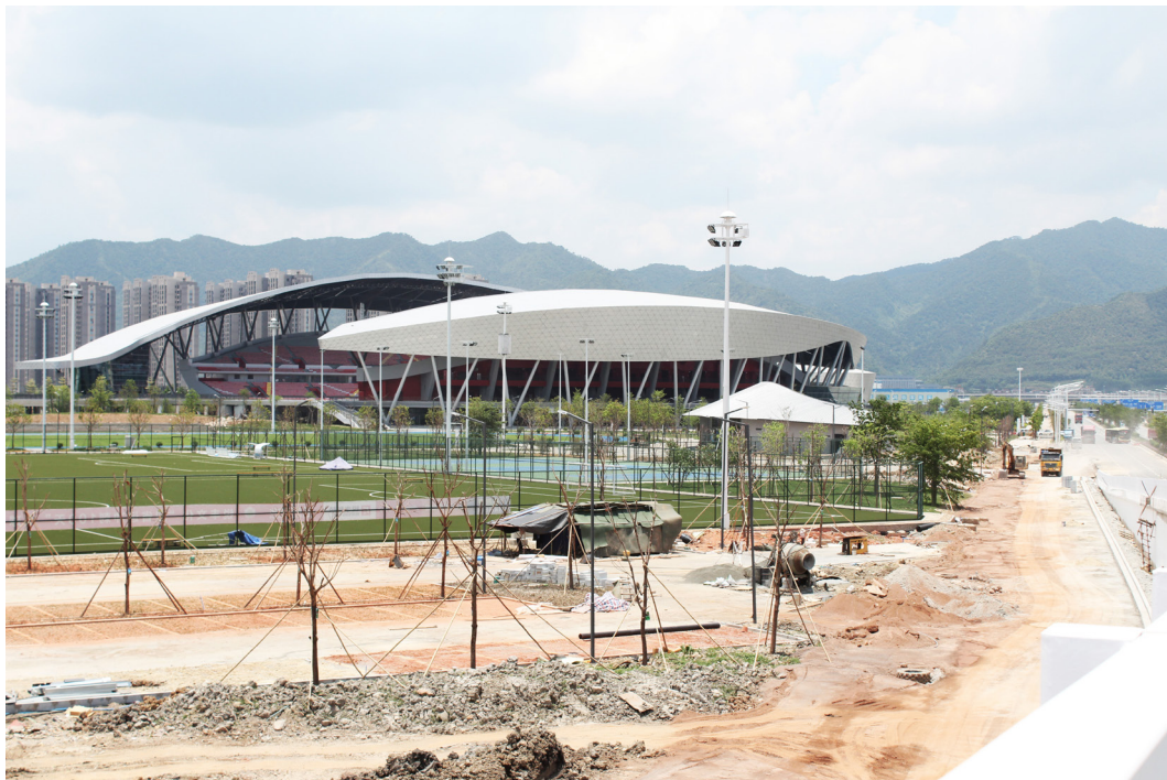
3.17 | Fully operational sport center within the construction site Zhaoqing New Area. Photo by the author. 2018
