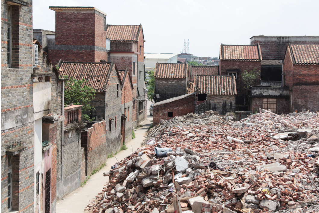
5.5 | Debris from the demolition of a rural village in Dinghu, Zhaoqing. Photo by the author. 2018
