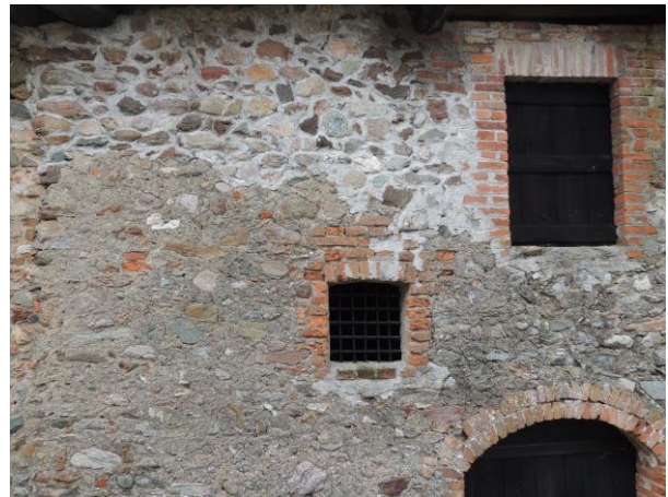
Figure 11. Building B - Reintegration of the masonry adopting inappropriate materials (credits Fabio Fratini).
