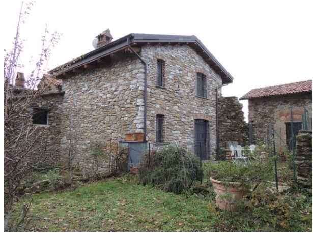
Figure 10. Building D - Reintegration of the upper part of the walls and of the roof (credits Manuela Mattone).
