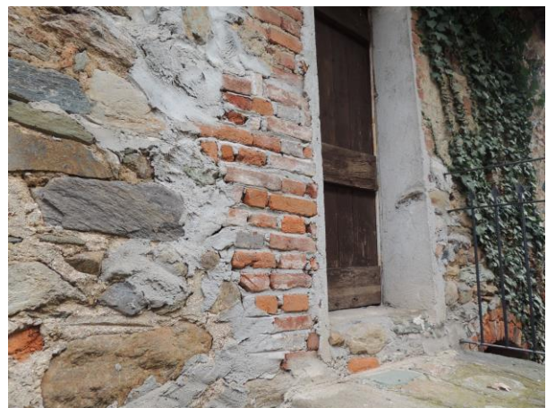
Figure 12. Building G - Improper intervention with cement mortar (credits Fabio Fratini).
