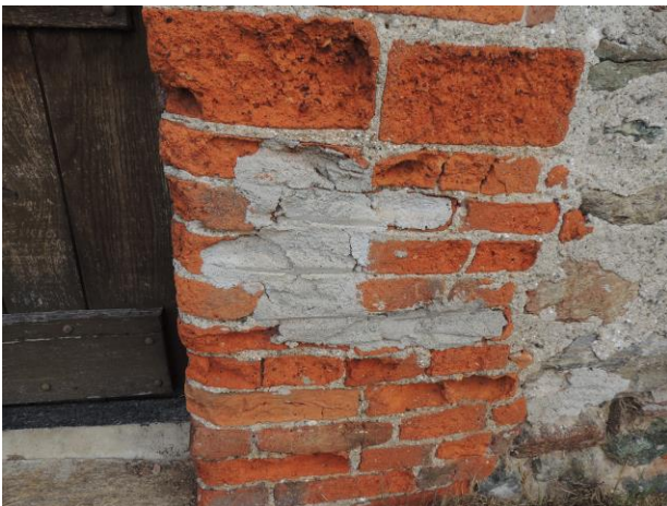
Figure 14. Building A - Reintegration of eroded bricks with cement mortar (credits Fabio Fratini).
