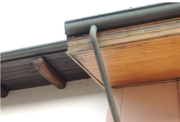
Figure 9. Building E - Wooden battens in the overhang of the roof (credits Fabio Fratini).
