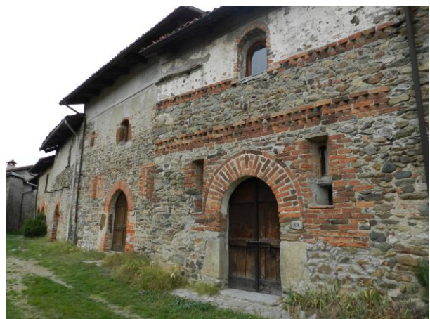
Figure 17. Building H - Preservation of the surface of the external wall and of the access portal (credits Silvia Rescic).
