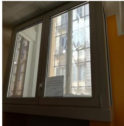
Figure 15. The new PVC window (on the front) and the original window (behind). Photo took on the ground-floor (the external window is shared with the mezzanine level). The sign asks to occupants to avoid operating the window due to the presence of mechanical ventilation.
