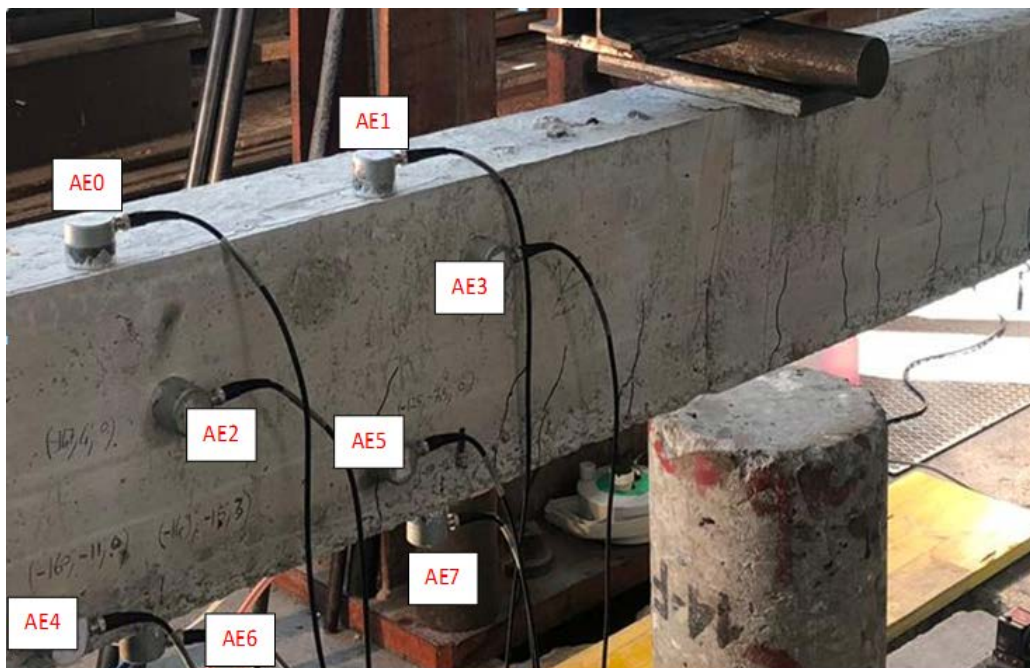
Figure 14. Crack pattern at loading step #7 and numbered AE sensors.
