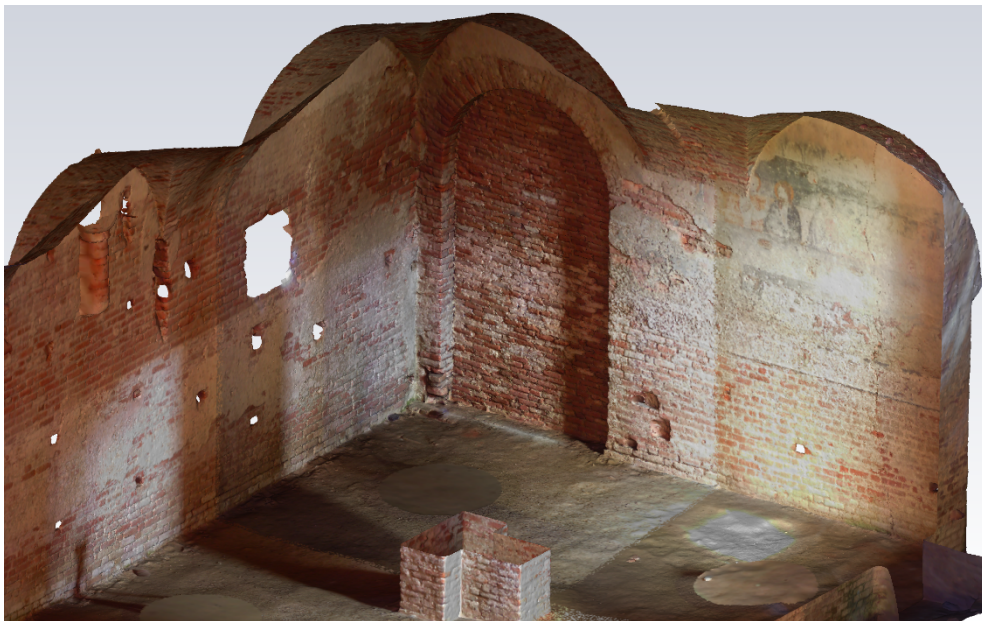
Figure 93. Radiometric values applied to the polygonal mesh (detail of south and east walls) - (elaboration F. Diara).
