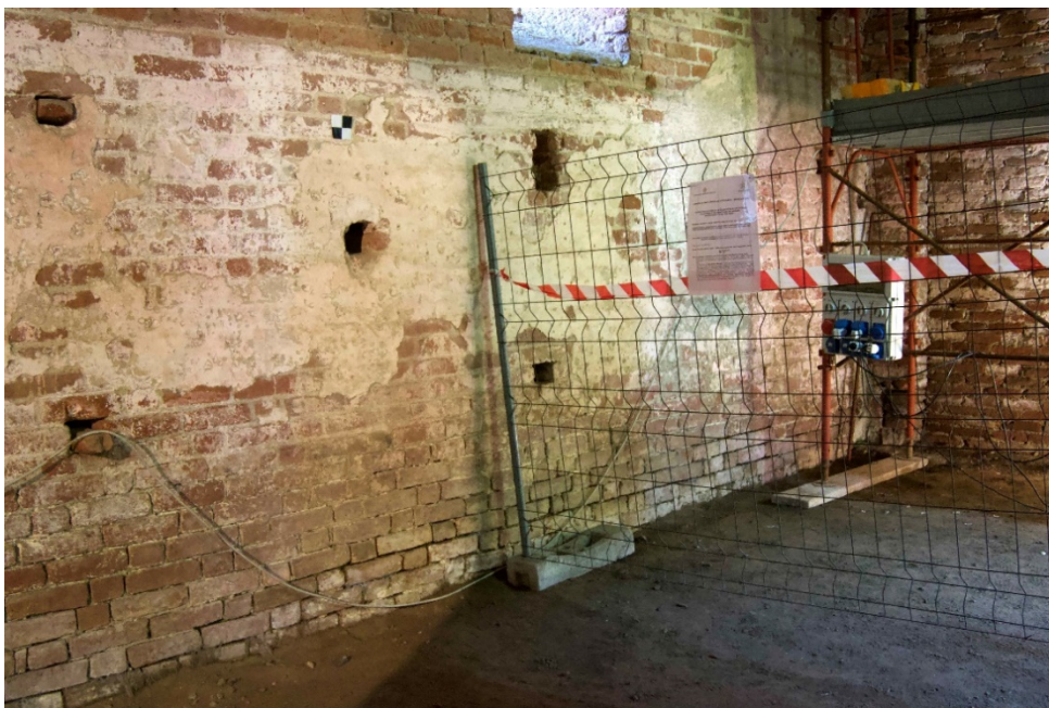
Figure 66. Image of north-east corner of the inner part of the refectory. On the right (east wall) can be noticed the restoration scaffolding (photo F. Diara)
