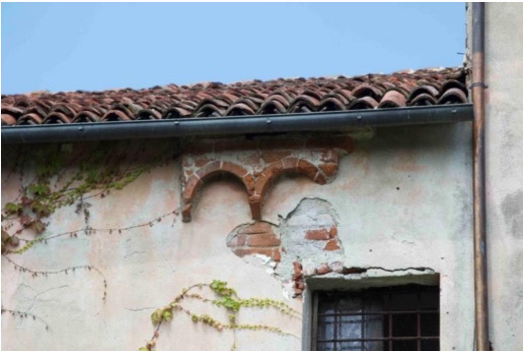
Figure 20. Evidences of protruding arches on the backyard side of the refectory (photo F. Diara)
