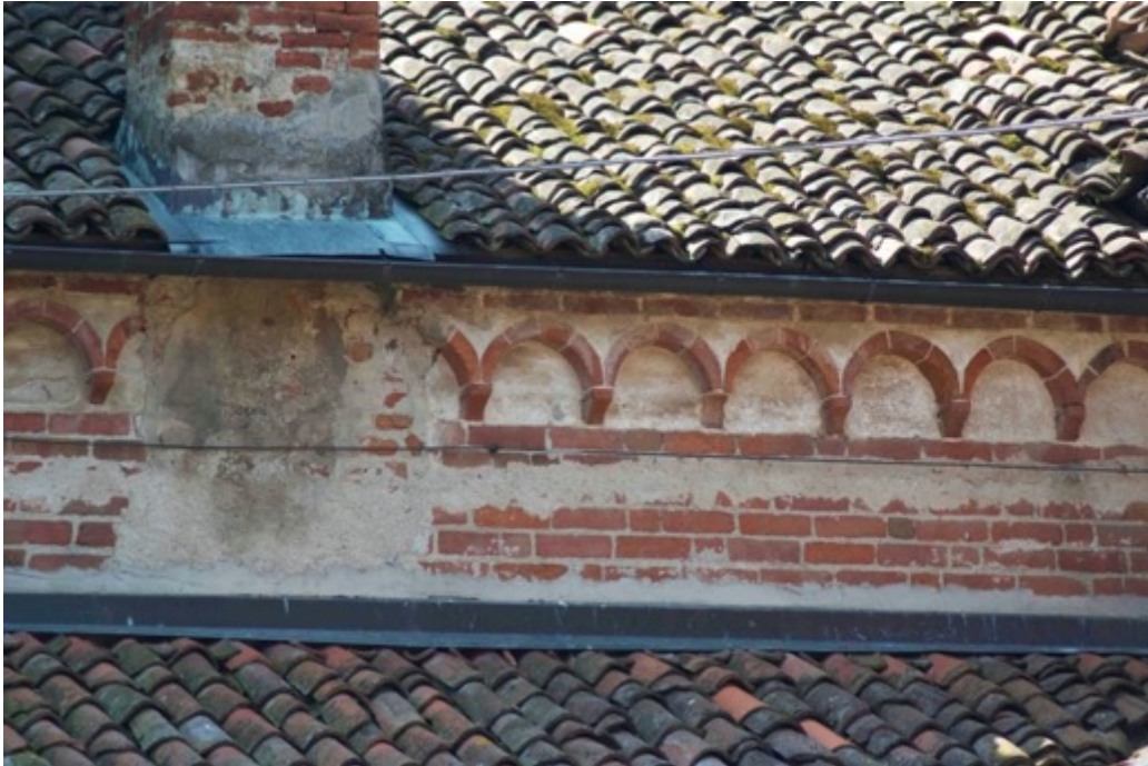
Figure 19. Protruding suspended arches on the external south front of the cloister, above the ceiling of gallery (photo F. Diara)
