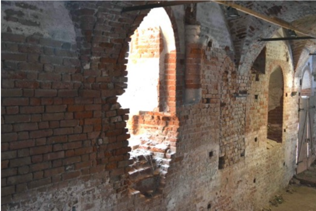
Figure 27. South wall of the refectory: detail of the removed pulpit and the window opened on its place; detail of the suspended semi column and a covered single lancet window (photo F. Diara)
