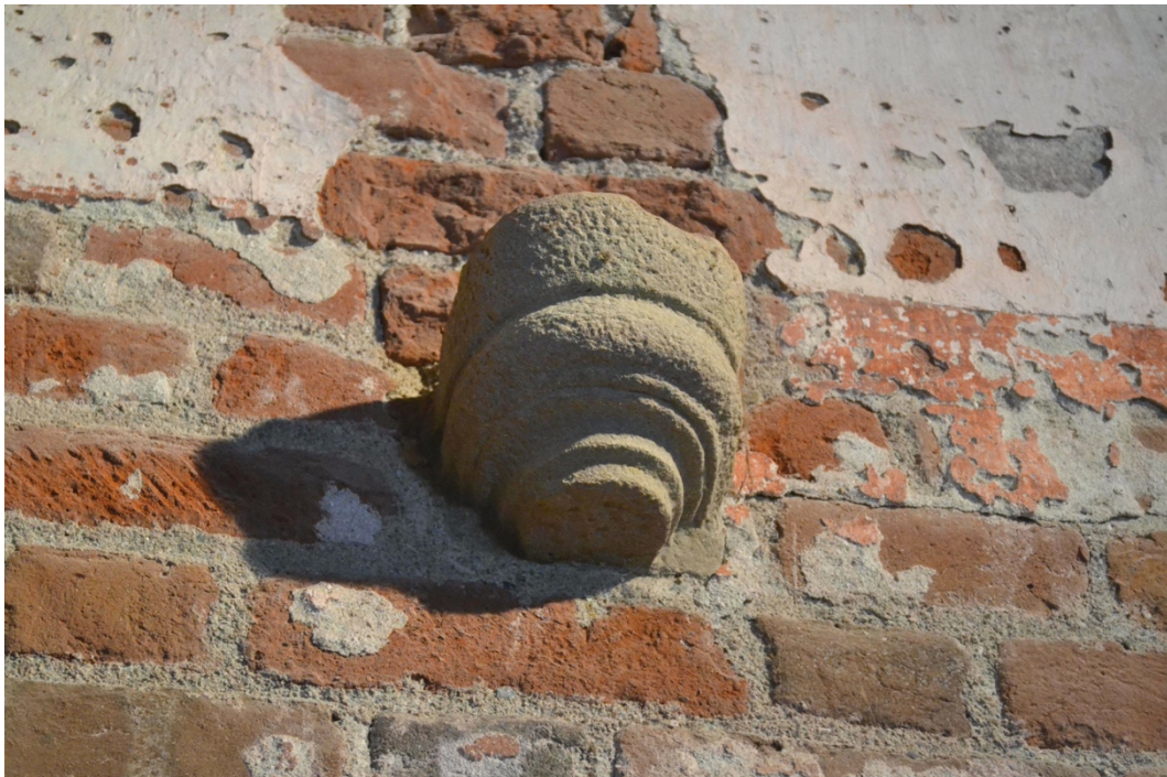
Figure 143. Detail of the stone shelf related to the old ceiling on the south wall of the refectory (Photo F. Diara)
