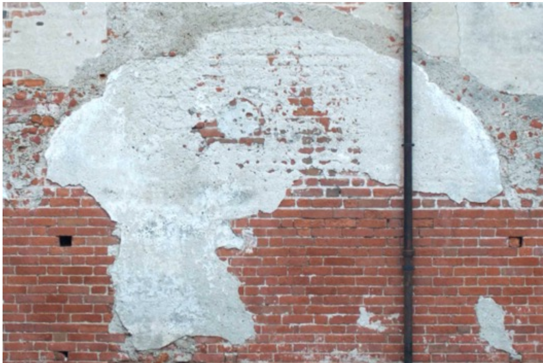
Figure 139. Detail of plaster and brick masonry with thin mortar joint on the south front of the cloister (Photo F. Diara)
