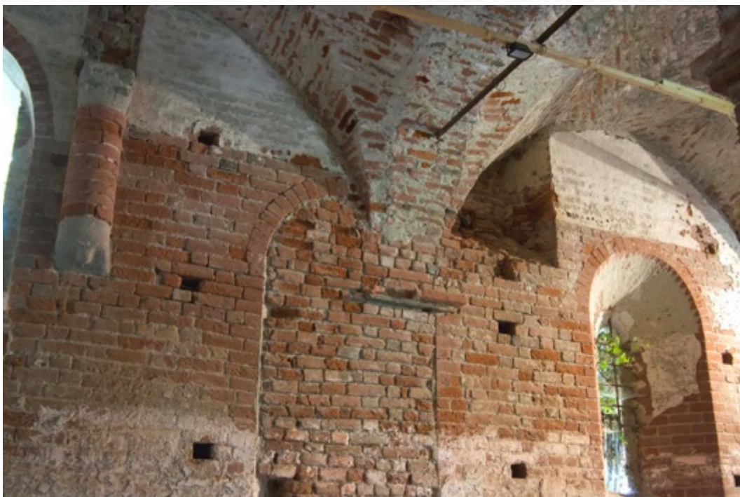
Figure 141. South wall of the refectory: can be noticed the walled single-lancet window (related to the opened one to the right) and the new vaulted system above it (Photo F. Diara)
