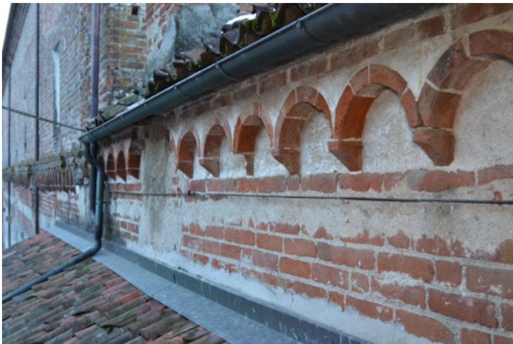
Figure 137. Suspended arches on the south front of the cloister (Photo F. Diara)
