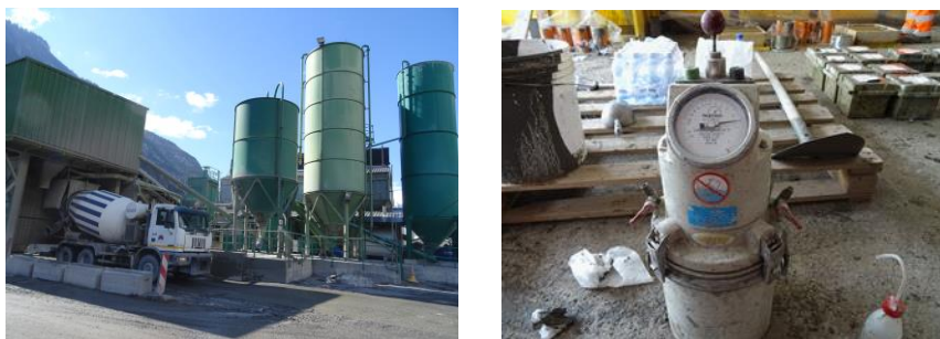
Figure 4.8 Production of SC-CBM at the batching plant (left) air content measurement (right)
