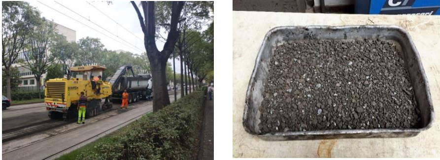
Figure 2.5 Milling of RAP from the pavement (left) and RAP used in the investigation (right)
