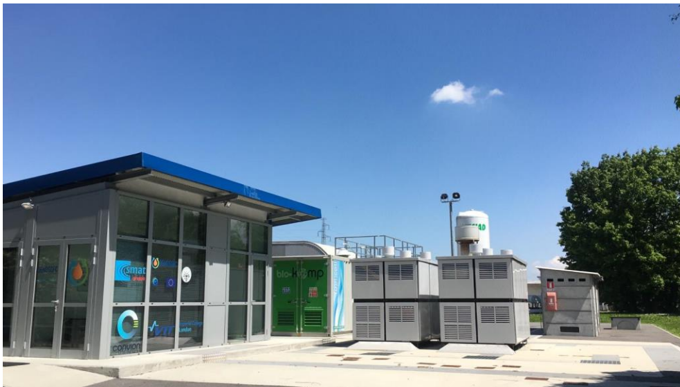
Figure 4. DEMOSOFC plant view. On the left, the technical building where the control room and the electrical cabinet room are located. On the right, the 2 SOFC modules. Between the control room and the modules, part of the biogas cleaning and compression container is also visible.
