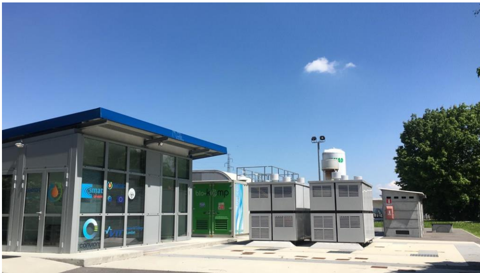
Figure 4. DEMOSOFC plant view. On the left, the technical building where the control room and the electrical cabinet room are located. On the right, the 2 SOFC modules. Between the control room and the modules, part of the biogas cleaning and compression container is also visible.
