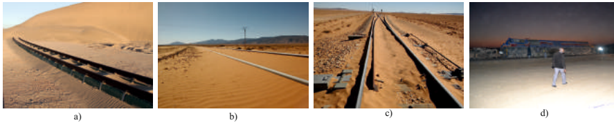
Fig. 2 Sand Ultimate Limit States: full coverage by encroaching sand dune (a, explicit publishing permission from the owner of the photo Giles Wiggs), partial coverage in a sandy plain (b), jammed turnout (c), train derailment (d, reprinted from [6] with the permission from the editor).
