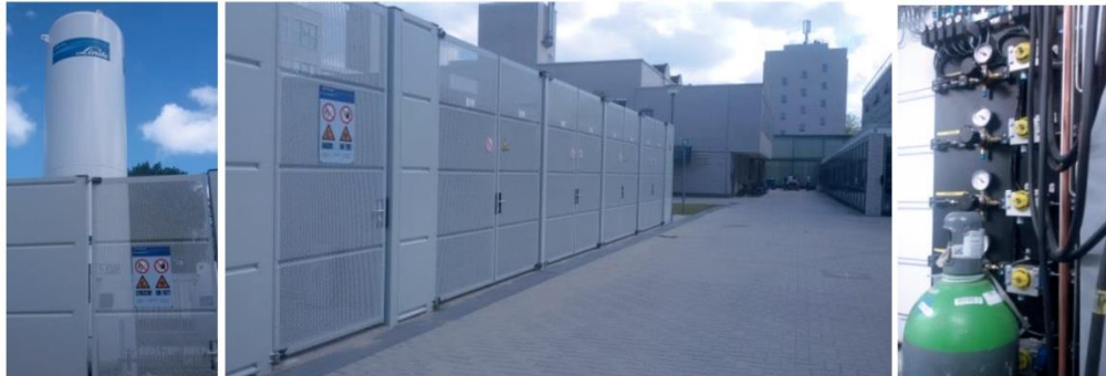
Gasses storage area and electric valves
