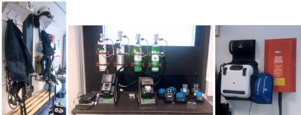
Detail of BHV equipment: PPE, gas detectors, initial control of fire equip.
