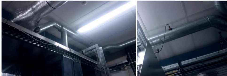
Flowrate sensor to detect possible failures in localized ventilation
