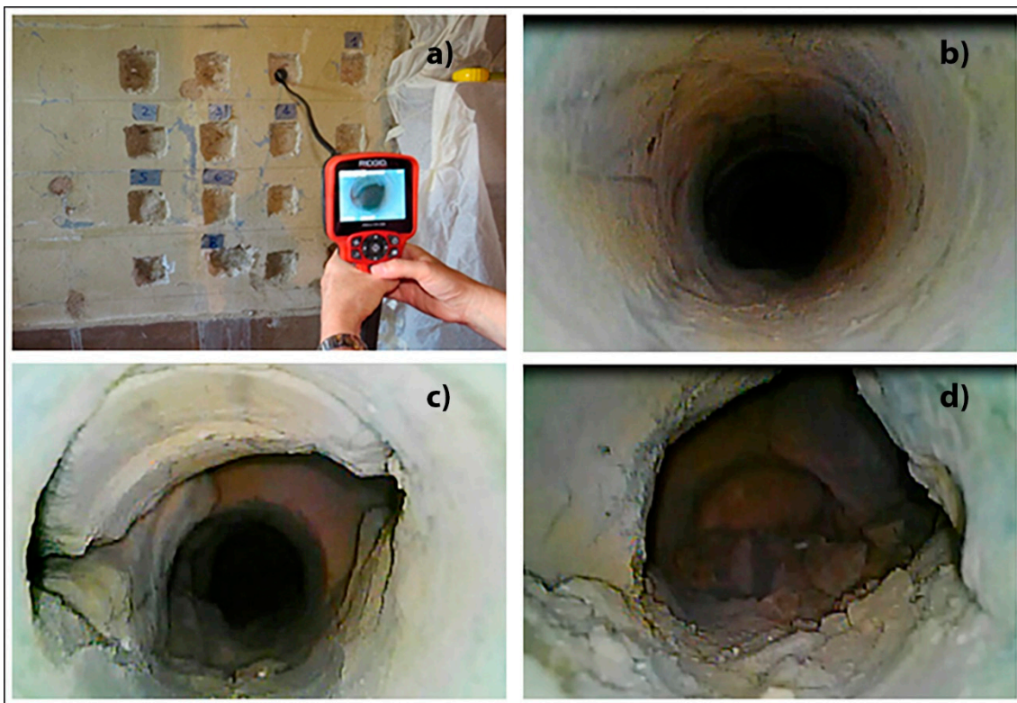
Figure 5. (a) Endoscopy surveys; (b) Initial section of compact masonry; (c) First discontinuity; (d) Central discontinuity between two walls.
