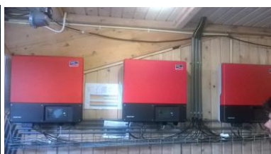
Inverters for the PV system
