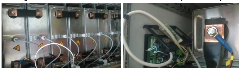
Li-ion battery (cells and BMS)
