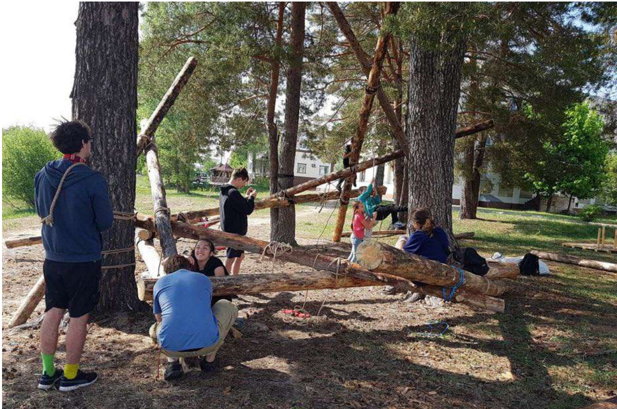
Figure 15: The construction site of Co-oCo-oNest prototype being built, used and re-designed by its users in the same time in Slavutych by Chernobyl, Ukraine. The project was to bring new futures speculations to, though by peoples' world attention abandoned, very rich developing new eco-system that is competitive to other ecological treasures of the world. The aim was to redirect the attention to the dead previously glowing past of the local community to the new opportunities of what the today's world issues bring. (photo: Davidová 2018)
