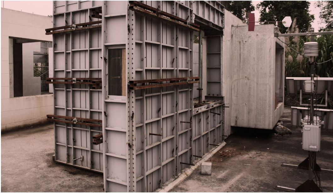
Figure 7.52: Aluminum forms for concrete casting in Vanke's Housing Industrialization Research Center in Dongguan (source: picture by the author).
