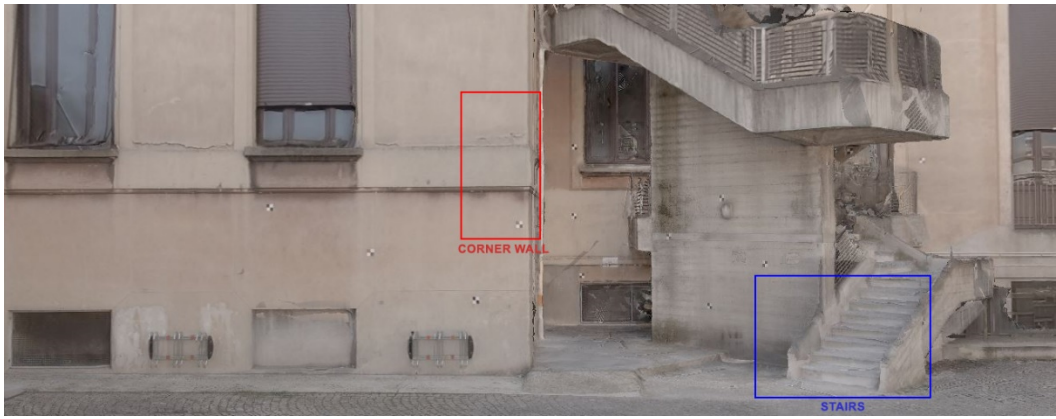
Figure 125 The two sample areas analysed: a corner between two walls and a portion of the fire stairs
