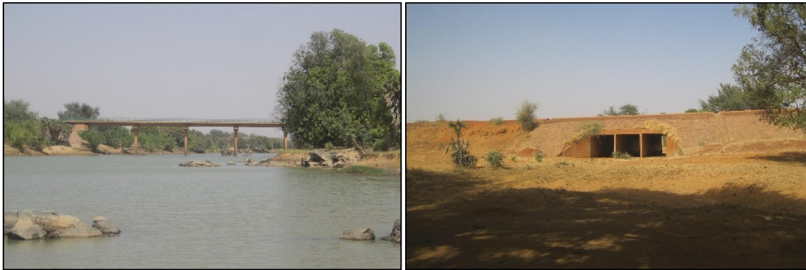
Figure 5. Left: The Farié bridge on the Sirba River. Right: the culvert with three opening placed on the left overbank.
