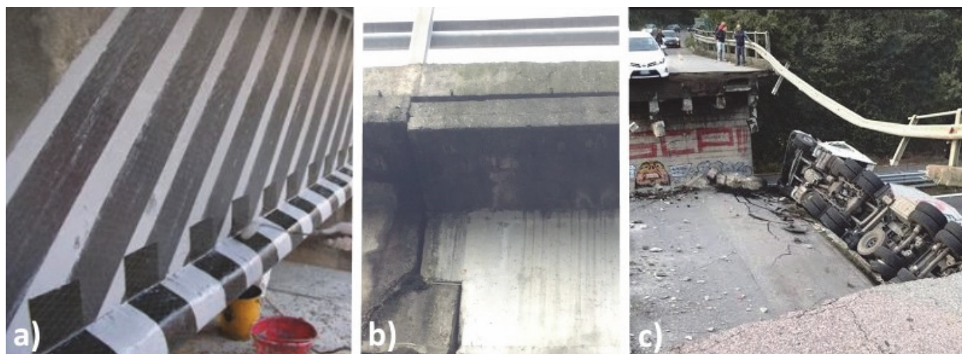
Figure 5: Dapped end corbel conditions before the collapse (a); humidity presence and water stagnation (b); failure loading configuration (c) [1].
