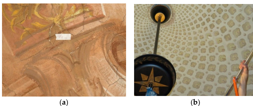
Figure 14. Points of potential plaster detachment: (a) P11 vault Pelagi room; (b) P15 vault Giunta room.
