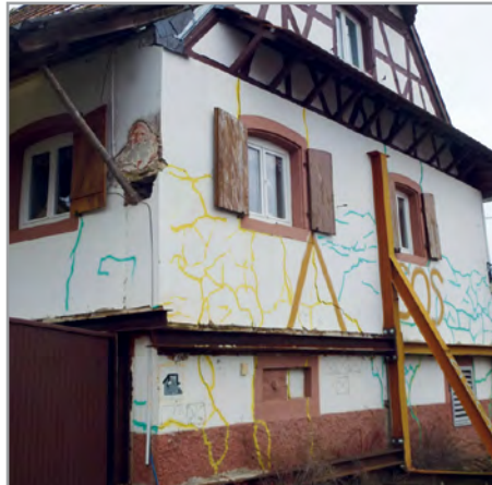
Houses affected by terrain movements in the village of Lochwiller (Alsace- France)
