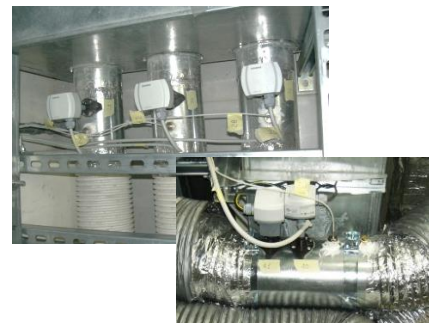
► Fig. 2: Part of the installed sensors in the mechanical ventilation system
