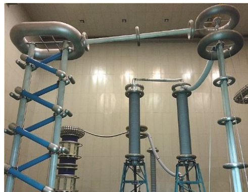
Fig. 14. \pm 500\text{kV} DC terminations under type test
