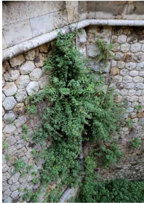
Fig. 4- Nitrophilous casmophytic vegetation ( Parietaron judaicae ) on the wall of Castello fortification realized with exagonal ashlar of limestone
