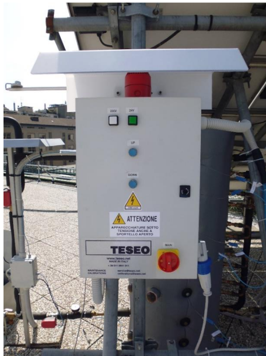
Figure 35. The electrical cabinet designed and installed to control the full-scale prototype.
