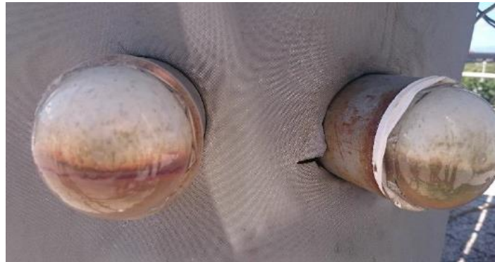
Figure 27. The thin layer of rust deposit affecting the inspection visors.
