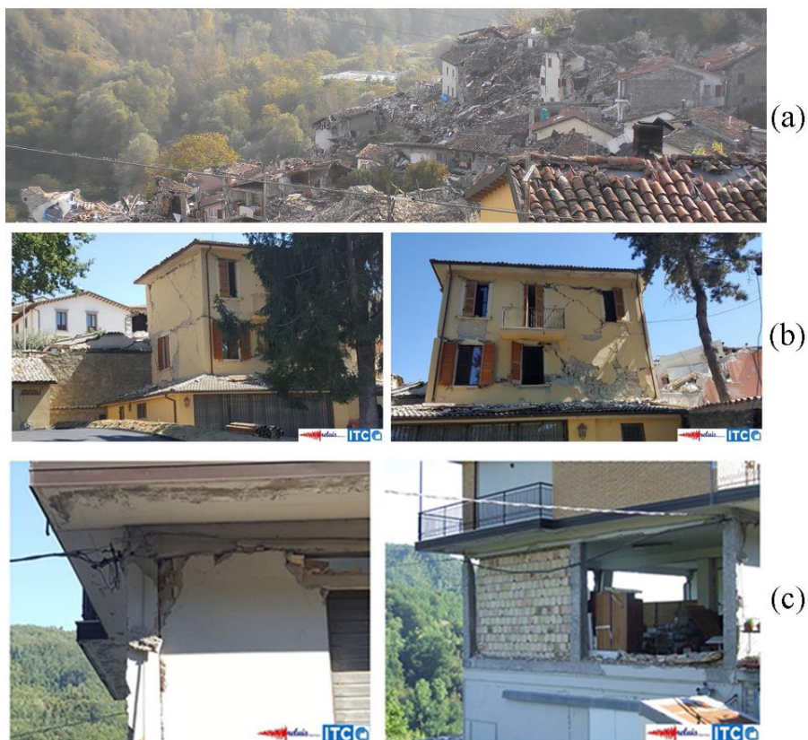
Figure 1.1: Effects of the earthquake in the centre of Italy in 2016: (a) Pescara del Tronto completely destroyed; (b) shear cracks in a masonry building at Amatrice; (c) plastic hinge and overturning of a masonry wall in a reinforced concrete building at Pescara del Tronto. (b) and (c) are images from (Celano et al., 2016).
