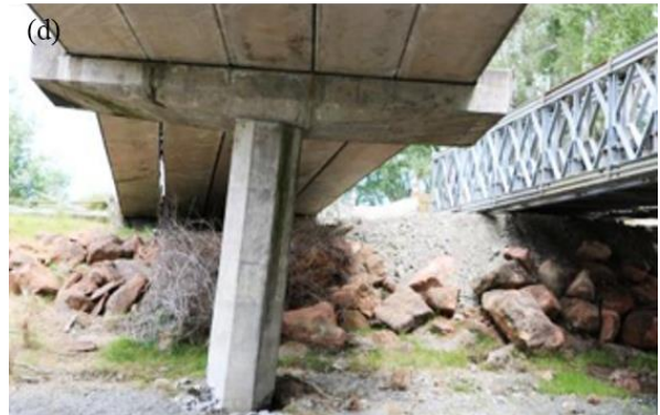
Lower Mason River Bridge; (c) Mason River Bridge; (d) Wandle River Bridge (Palermo et al., 2017).
