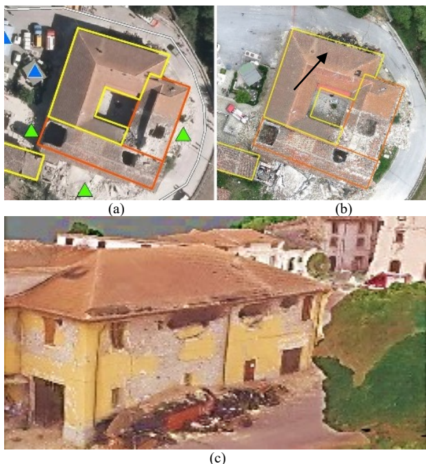
Figure 11. BDA on Accumoli site, in a sample building. The aerial image of Copernicus (a), the UAVs orthophoto (b) and a view of the considered damaged façade in the 3D model inspection (c).
