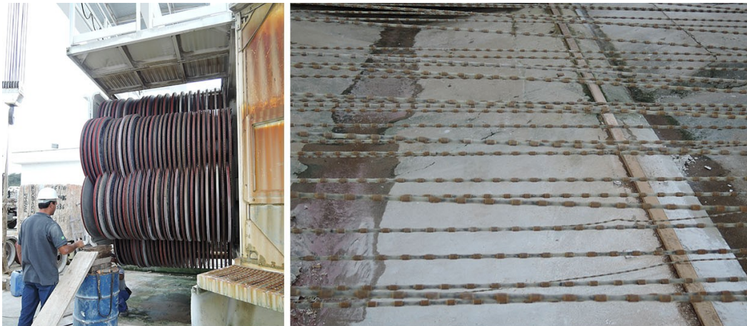
Figure 25: pulleys and diamond wires installed in a diamond multi-wire cutting machine
