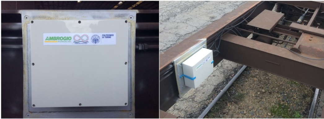
Figure 29. Central monitoring systems installed on steel plate.
