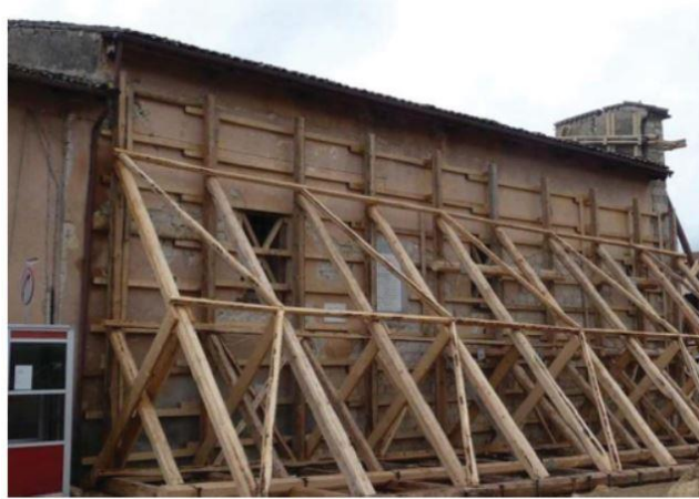
Figure 20: propping intervention of lateral wall of church of Onna (AQ). Source (Modena, et al., 2011).
