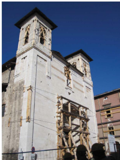
Figure 21: shoring of facade with cables and wooden frames (Chiesa di S. Marco, L'Aquila). Source (Modena, et al., 2011).
