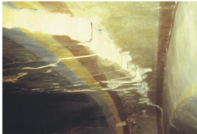
Figure 32: cracks and deformation in the vaults with relative displacement till 30cm. Source (Crocì, 2000).
