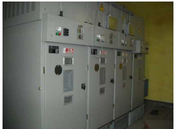
Fig. 5. MV switchgear in the faulted substation.
