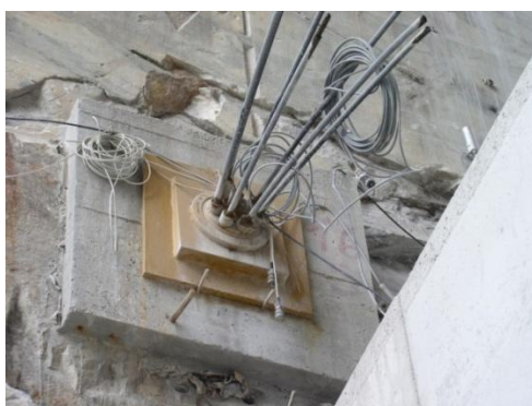
Figure 3. Instrumented tendon head on the left wall of the cavern: an anular load cell at the tendons head with a tiltmeter.
