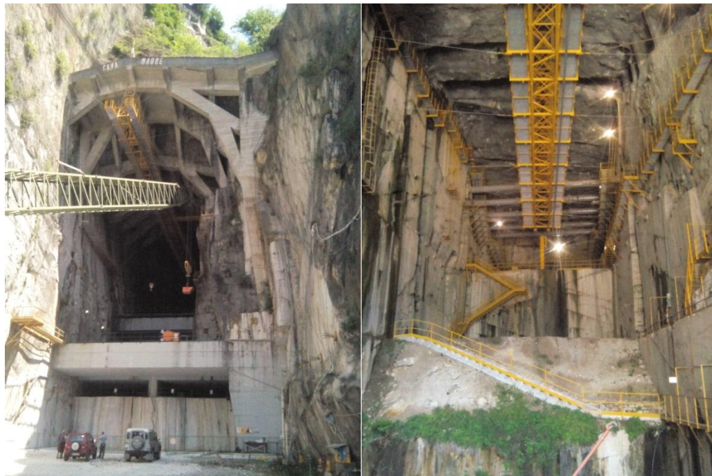
Figure 1. Left: The adit of the Candoglia Cavern, where the marble exploitation is now developing. Right: The inner zone of the Cavern, where the mining activity is now abandoned.
