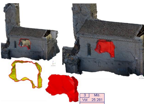
Figure 12. Analysis on West wall where the damage mechanisms caused the collapse of the central part of the masonry by shear failures.
