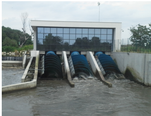
Fig. 1.8. Archimedes screw used as turbine. Three installations in parallel (picture of Quaranta, 2016).
