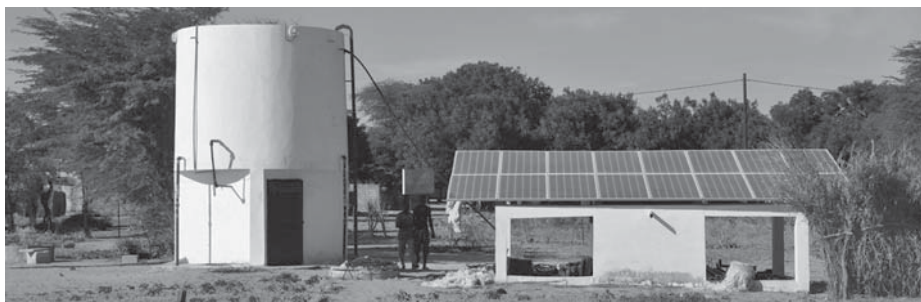
Figure 11.4: The solar platform of village, Ndia (Photo by the author, 2013)
