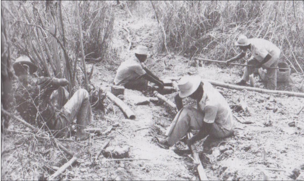
Figure 39: Construction of water supply system having bamboo as raw material - Juramento Project of Alternative Technology. In Moraes (2006).
