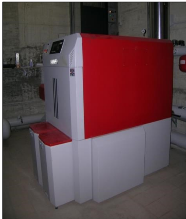
Figure 4.7 – Example of analyzed chips boiler
