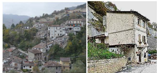
Figure 1. Pescara del Tronto perched village, in Arquata del Tronto, AP, October 2016 (left). The object of focus: a stand-alone damaged building (right).
