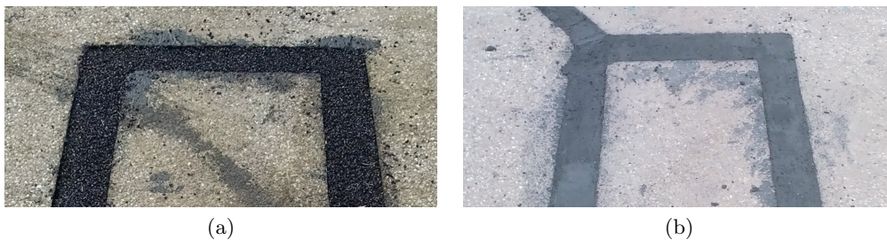
Figure 7.27: Appearance of the hole filled with cold asphalt (a) and MAPEI Mapegrout (b).
