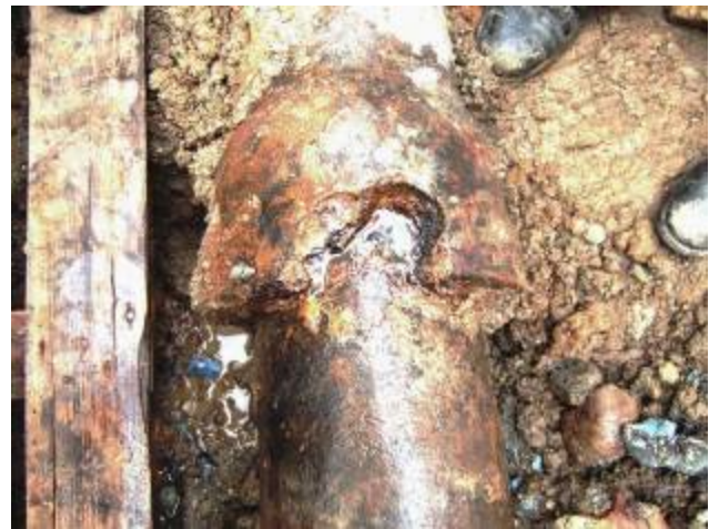
Fig. 7 – Water pipe damage
