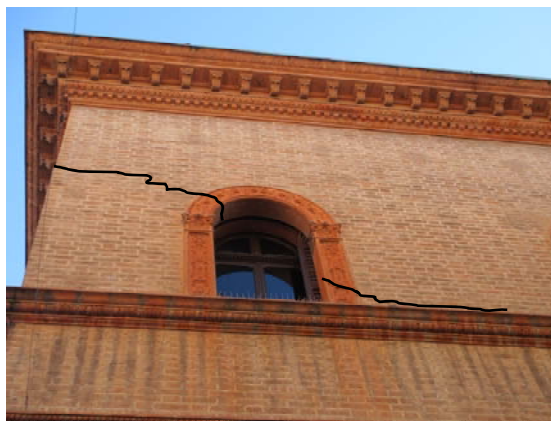
Fig. 4 Diagonal cracks on external windows
