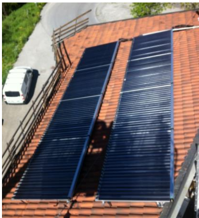
Figure 6 – ETC installed on the roof
