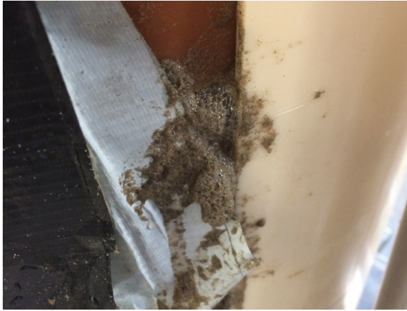
Figure 7.57: Broken membrane with the foam flowing out from the sample (drained conditions).
