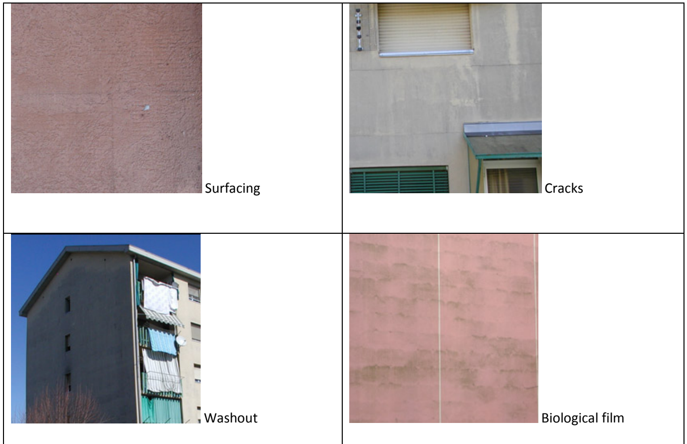
Fig 2: The main defects considered in the study.
